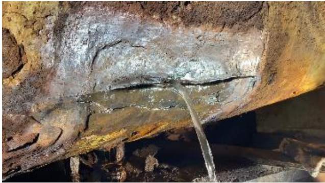
(Fig 1) Active Leak on a 54" saltwater Intake. Cracked pipe with a 1.5" hole. Extreme Corrosion.
