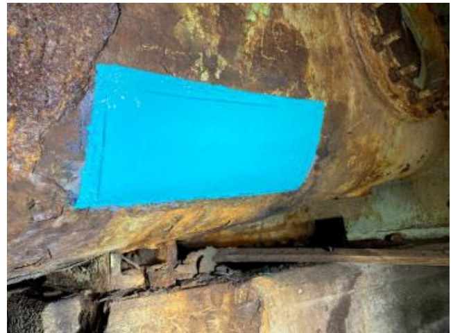
(Fig 4) - A top coating of RUBBEREX Epoxy Liquid applied to steel plate for protection from corrosion.
