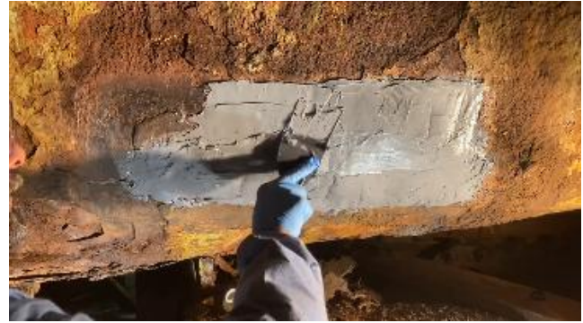
(Fig 2) - Active Leak Stopped by LEAKLOX Epoxy #403 Followed by Industrial Metal w/Fiberzite Reinforcement
