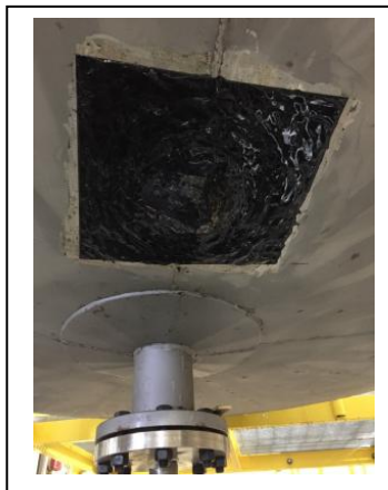
Tank Leak/Corrode weld. Leaking tank repaired with TANK REPAIR EPOXY.
